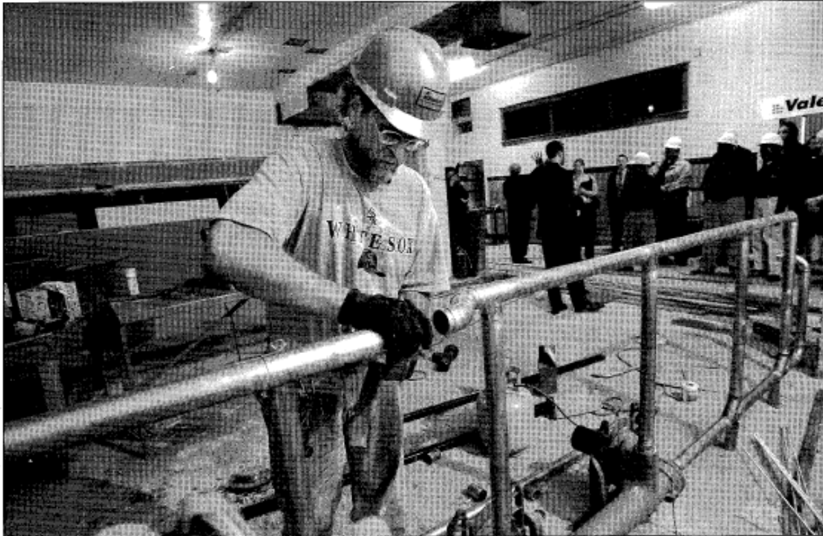
Chris Lodygowski works on the plumbing at the former home of St. Martin de Porres Grade School, the future home of Chicago Jesuit Academy. The Jesuit middle school has shown great progress in helping pupils from poor neighborhoods.
